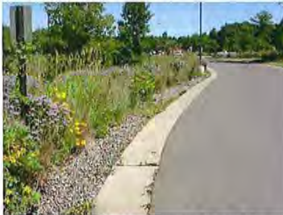
Figure 29, sub-surface infiltration bed with vegetation.
