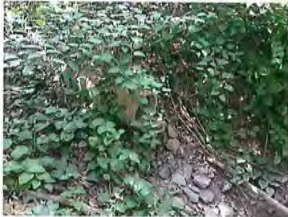
Figure 12, view of stormpipe outfall and eroded streambank.
